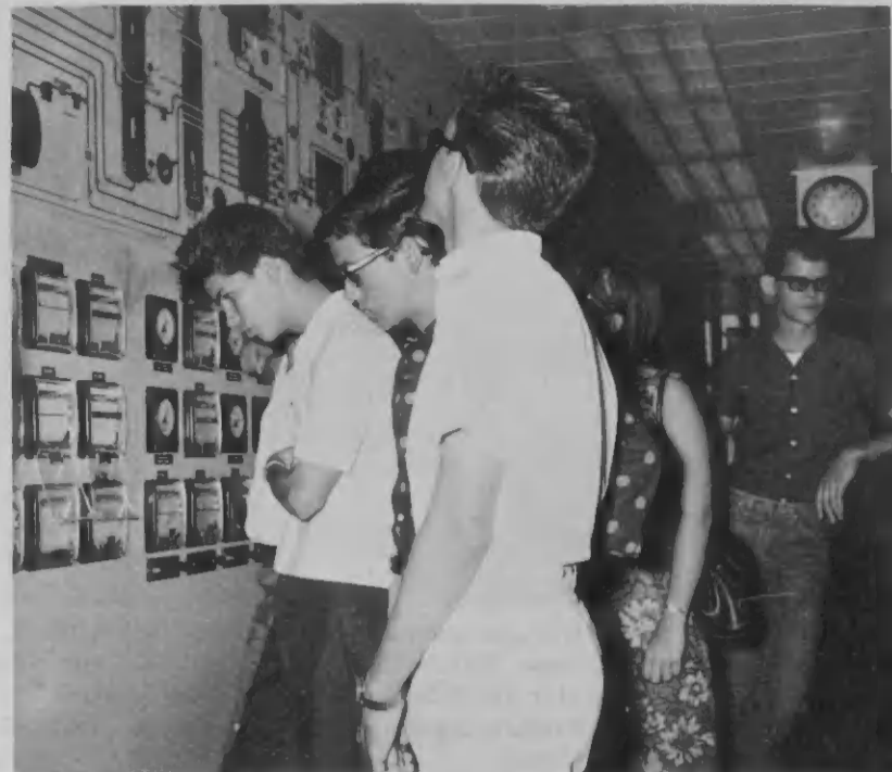
ST. ANTONIUS COLLEGE students observe combination unit control panel during their refinery tour. ESTUDIANTES DI Antonius College ta observa panel di control di Combination Unit durante nan tour den refineria.
